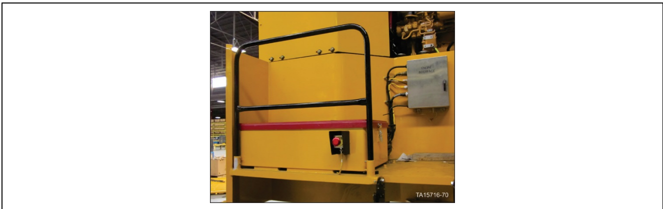
Figure 1. Battery box location
